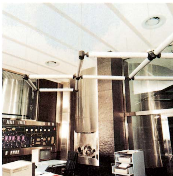
Control room: König Brewery, Duisburg
